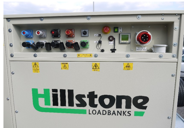
Typical control panel and cable connections
